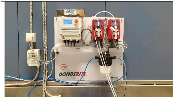
Fig. 1: Automated dosing of degreasing agents
